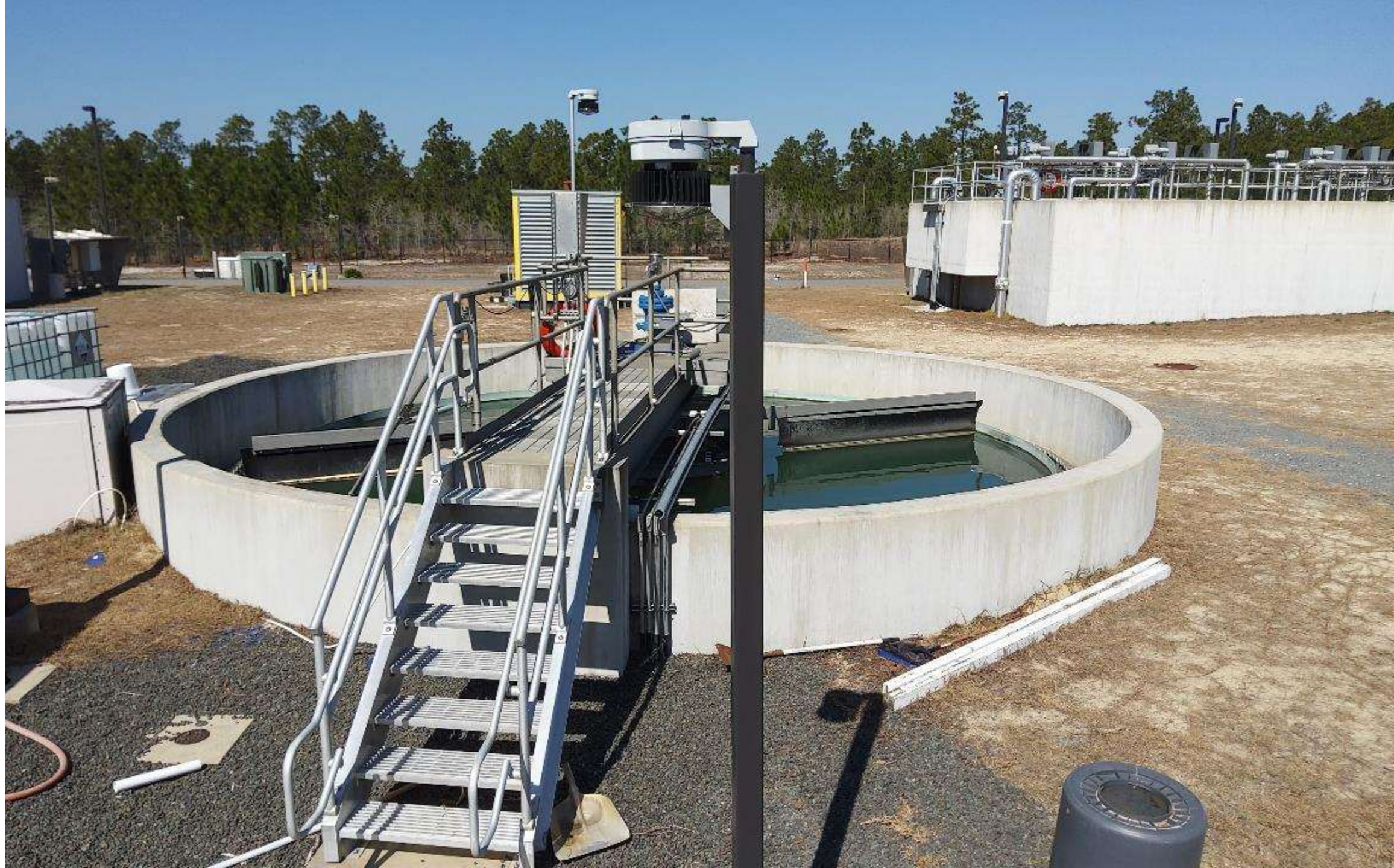
A View of secondary clarifier 1 with the MBBR in the background (right).
