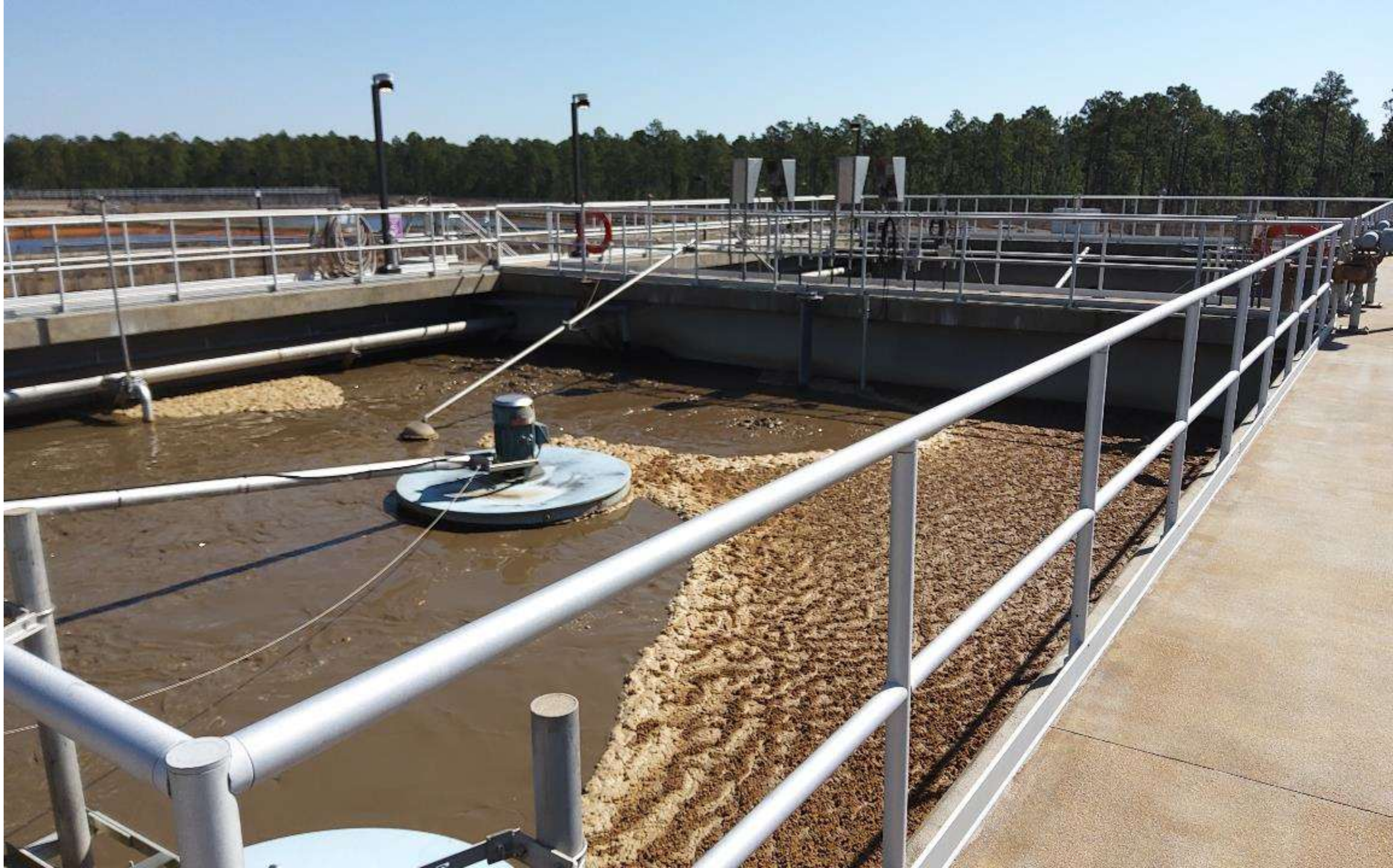
A View of the aerobic digesters.
