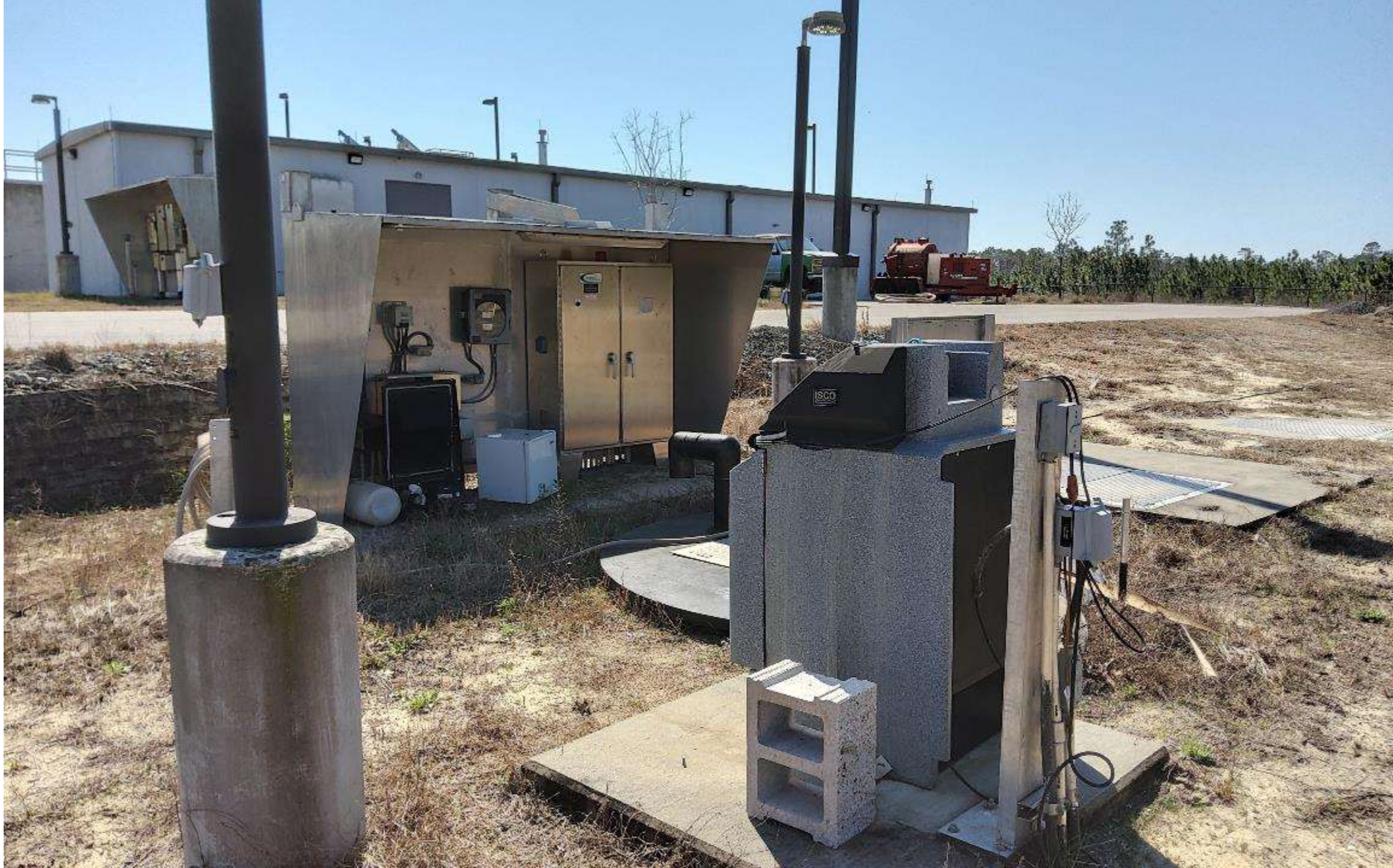
A View of the influent pumping station
