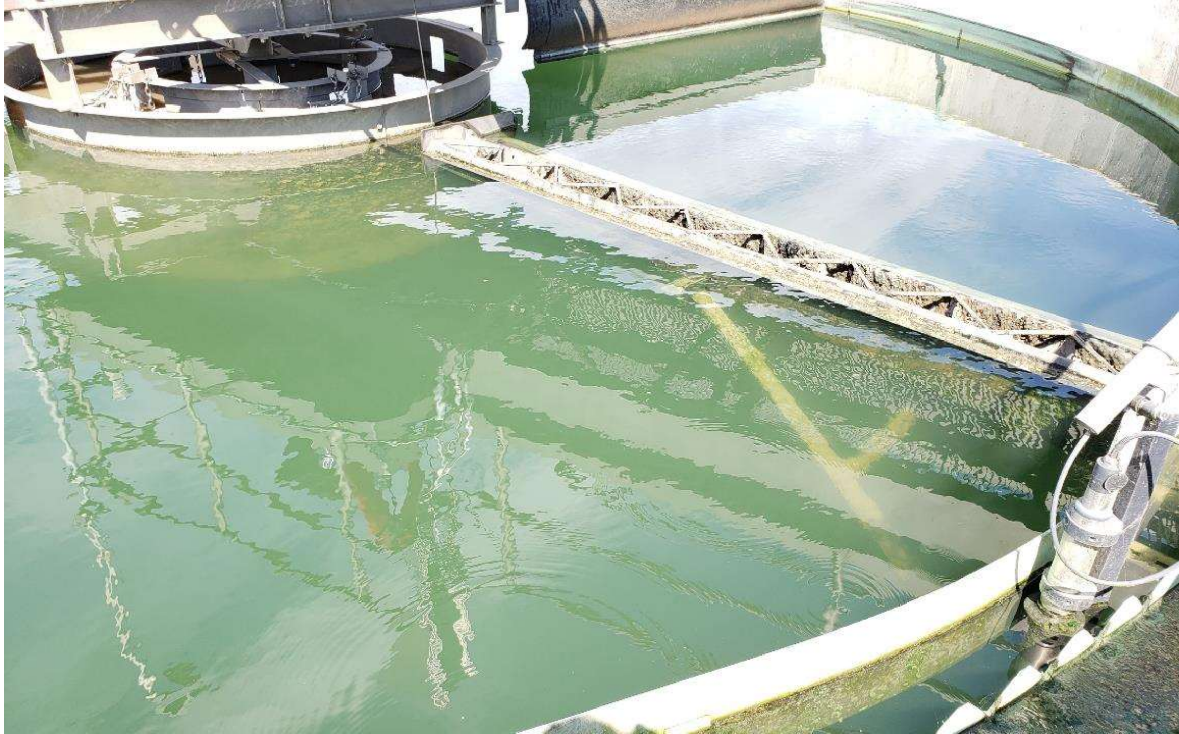
A View of secondary clarifier 2.
